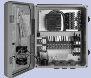
MVP-SSF Series Sand Filter Control Panel
