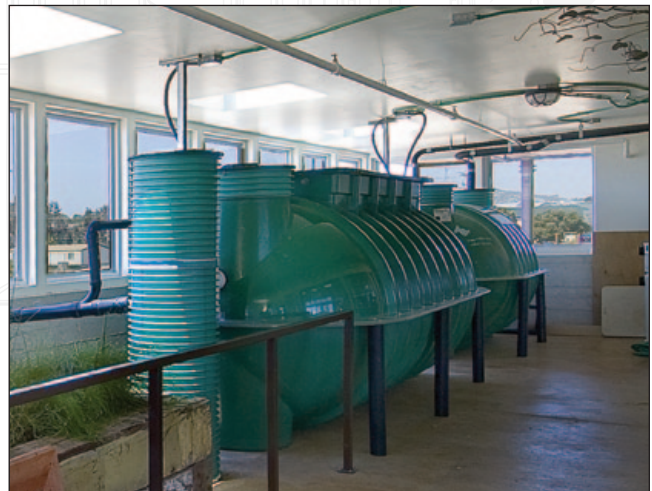
The off-the-grid EcoCenter at Heron's Head Park in San Francisco includes an above-ground, indoor AdvanTex Textile Treatment System followed by a constructed wetland and UV disinfection. Treated water is recycled for landscape irrigation. The U.S. EPA honored the EcoCenter with its 2010 Environmental Justice Achievement Award.
